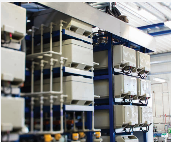
AFC Energy's 240kW fuel cell system, the world's largest AFC installation, at our plant in Stade, Germany.
