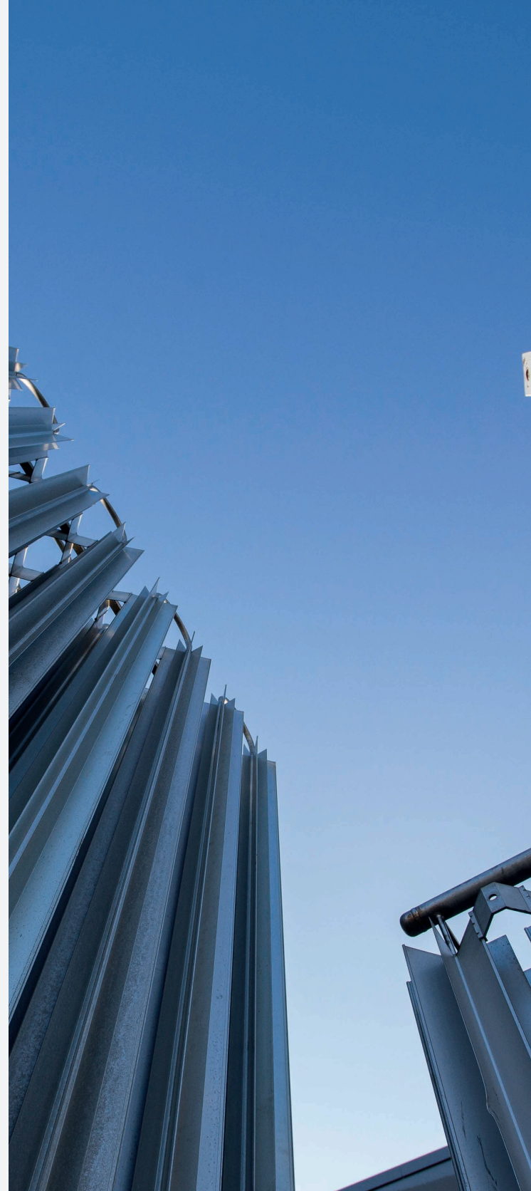
Liquid nitrogen tanks and evaporators.
