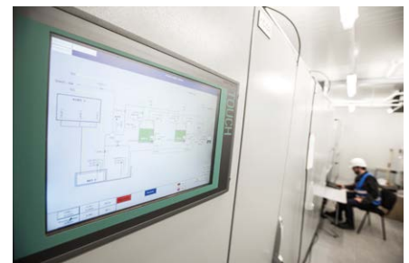
Control Panel for the Distributed Control System
