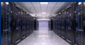
Datacentres and buildings for emergency back-up power
