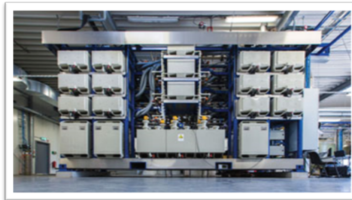
AFC Energy 240kW Alkaline Fuel Cell System Installed in Stade, Germany
