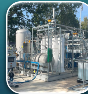
Hydrogen Production - Ammonia Cracker
